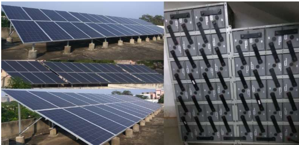
(Solar panels at NCDS)
